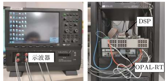
图 13 半实物测试系统图 Fig.13 Hardware in the loop test system diagram
